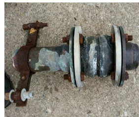
Failed Expansion Joint for Domestic Hot Water
