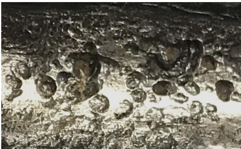
Figure 7: MIC attack and hole in 2 3/8" tubing experienced in downhole environment of Midland Basin Wolfcamp well (189-days after completion). 15
