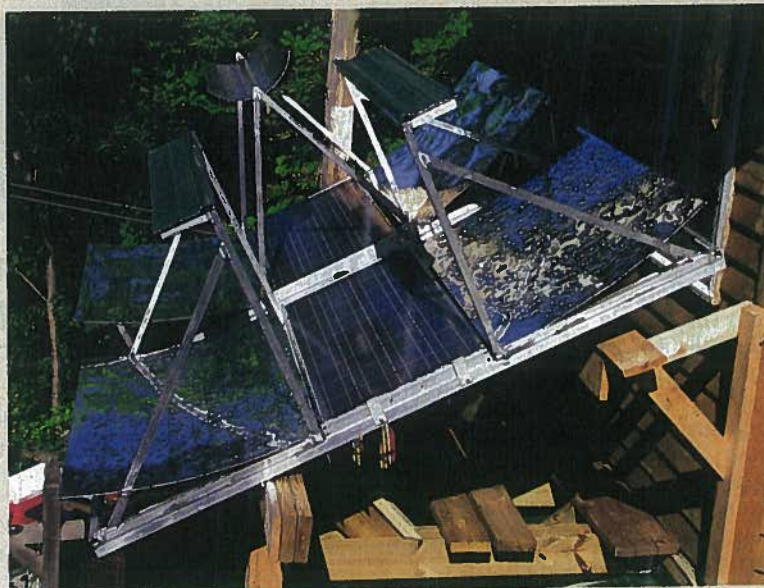
Parabolic reflectors gather three times the typical sunlight for PV panels, boosting electricity generation and creating excess heat that is captured for heating.
