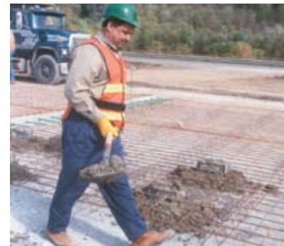
Shad Sargand, Russ Professor of Civil Engineering and assistant director of ORITE, carries concrete to fill strain-gauge boxes prior to placement of concrete on US50 East in Athens.
