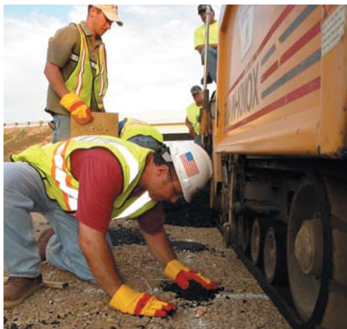
Preparing for later measurement of strain due to traffic load, ORITE Research Engineer Issam Khoury and civil engineering graduate student Michael Romanello install asphalt strain gauges on US30 in Wayne County.
